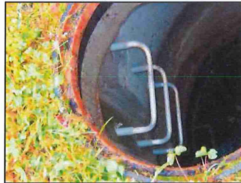
Photo 30: Pugsley lift station manhole
