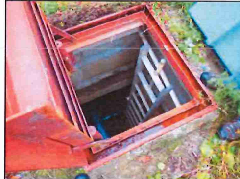
Photo 7: Waterfall Creek valve chamber
