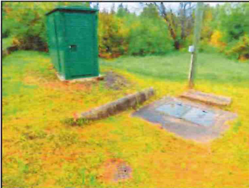
Photo 32: Bowser lift station
