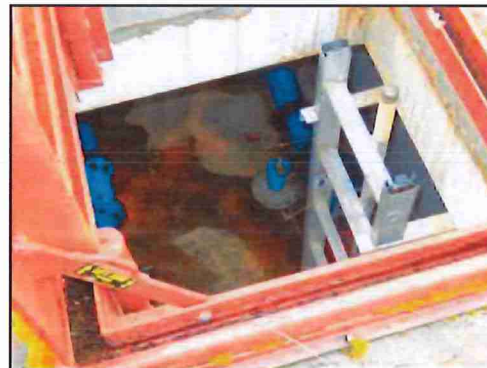
Photo 17: Reservoir valve chamber
