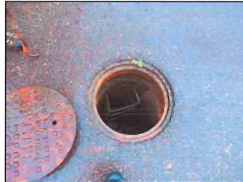
Photo 33: Bowser lift station manhole
