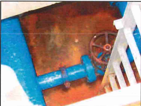
Photo 8: Waterfall Creek valve chamber
