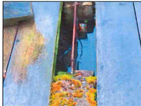
Photo 35: Lagoon discharge weir
