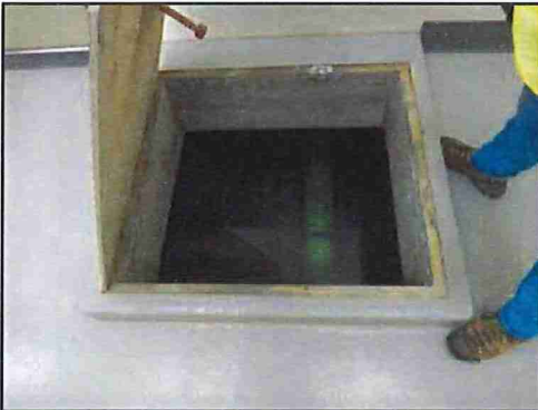
Photo 13: Contact chamber access
