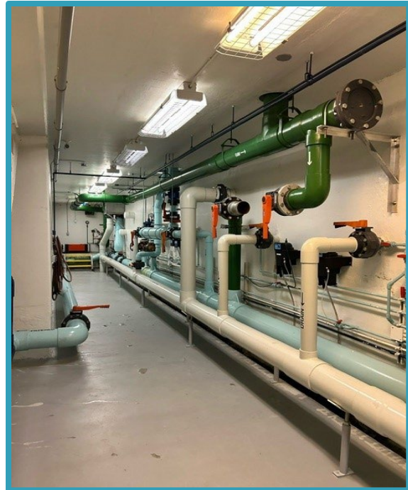
The inside of our water treatment plant, look at those pipes!
